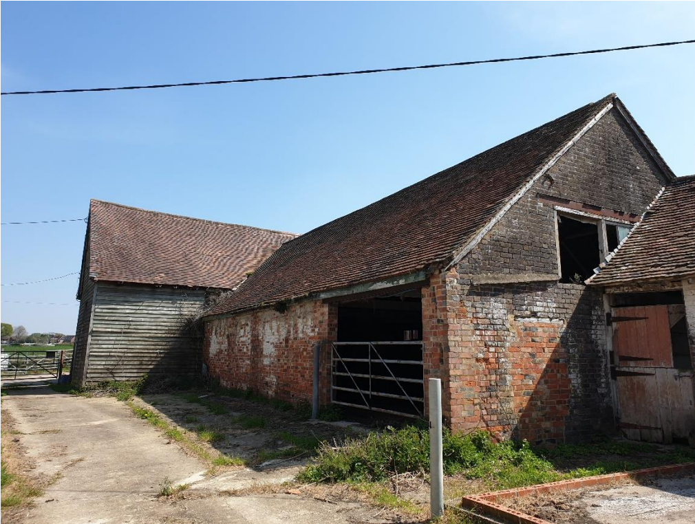
Figure 20: Barn B, with brick masonry and tile covered roof, late nineteenth century.
