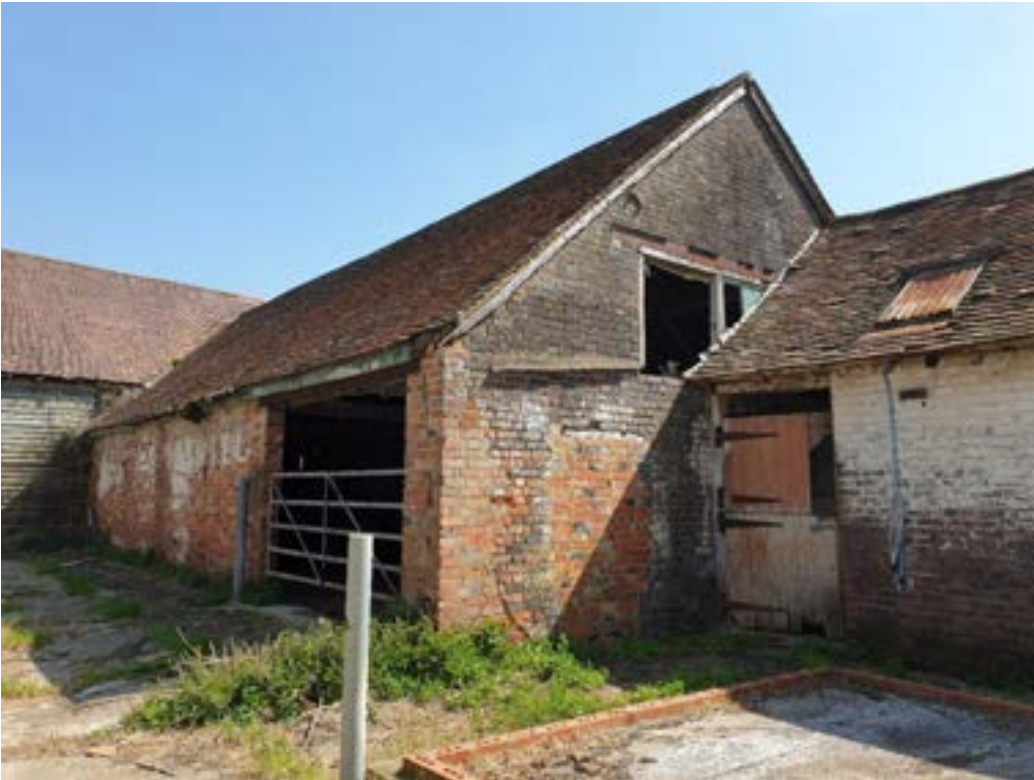
Figure 20: Barns B and C, Barns at Great House farm in 2022, identified as a non-designated heritage asset.
