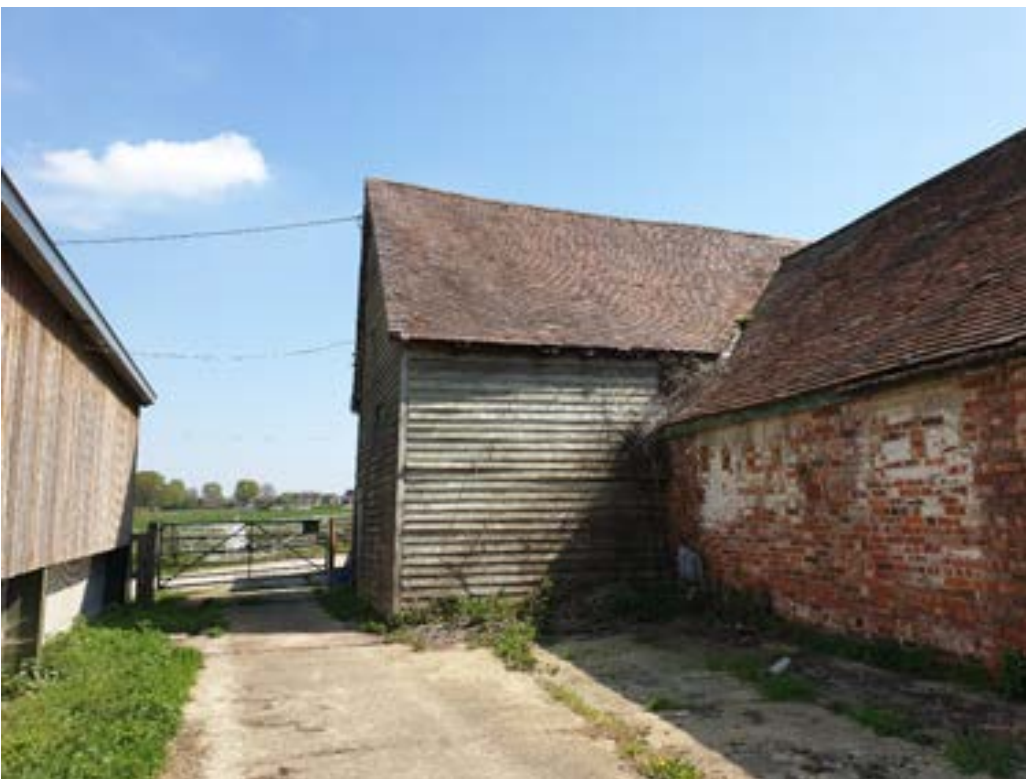
Figure 19: Barn A in 2022, Barns at Great House Farm, identified as a non-designated heritage asset. Further deterioration has taken place since this image was taken.
