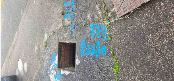
MH22X_85d67e76-ba9a-4451-bc9d-5637e654a12e_20241125_100811.jpg, 00:00:03, 0.00 m General remark, LINE HOLDING, MH24 REQUIRES EMPTYING
