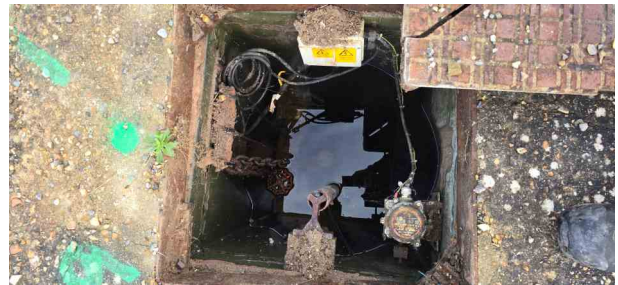
MH32X_6476d4ac-80fb-4081-a5f3-cf29dca6fb3d_20241125_112757.jpg, 00:00:55, 14.78 m Finish node, manhole, reference: MH32, PUMP IN CHAMBER, NOT WORKING
