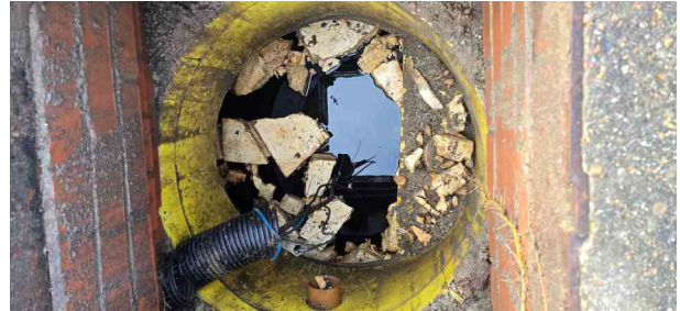
MH23X_b2a02f52-d2a0-40f8-8de7-244e290f80c2_20241125_100934.jpg, 00:00:03, 0.00 m General remark, INTERCEPTOR REQUIRES EMPTYING TO SURVEY
