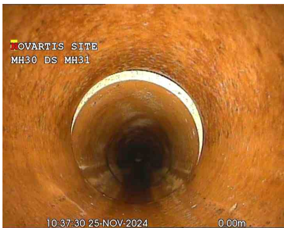
MH30X_be1fa4e2-0bad-4938-8c7d-66491d64b79e_20241125_104944_019.jpg, 00:00:10, 0.28 m Joint displaced, large
