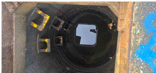
MH23X_6dcffdca-c3d8-4f4e-adff-02b165a218c5_20241125_100841.jpg, 00:00:03, 0.00 m General remark, INTERCEPTOR MH24 REQUIRES EMPTYING TO SURVEY
