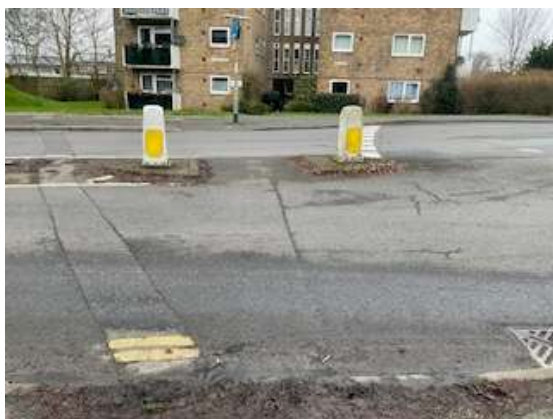
Figure 2: Ponding and detritus at crossing point.
