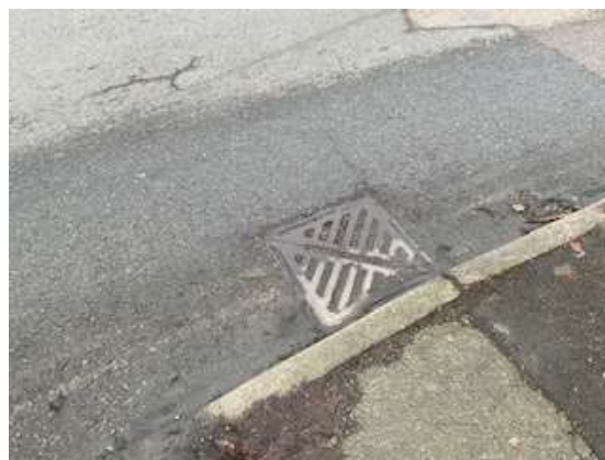
Figure 3: Blocked gully to the northeast of the crossing point.
