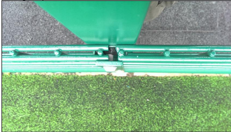
Figure 9: Image showing neoprene isolators
