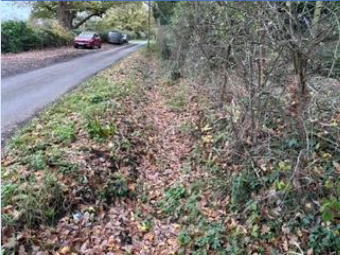
Figure 6: Ditch along Mayes Lane to the South of the Footpath (Source: Robert Sharpe)
