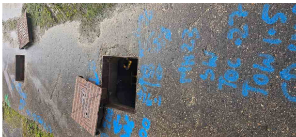
MH23X_7e7af6c9-528c-478b-9e05-63c4d5869097_20241125_100835.jpg, 00:00:03, 0.00 m General remark, INTERCEPTOR MH24 REQUIRES EMPTYING TO SURVEY
