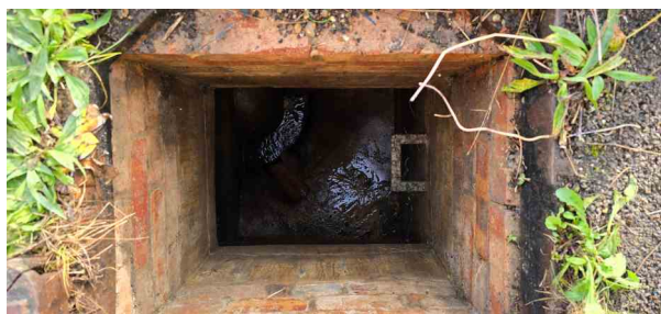
MH31X_a5845c64-2fc7-405d-9f44-63ba8d392b8f_20241125_104917.jpg, 00:01:07, 14.10 m Finish node, manhole, reference: MH41
