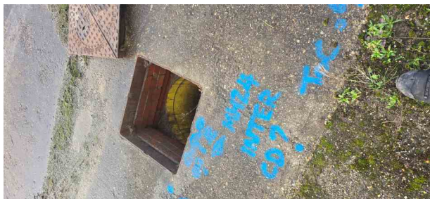
MH23X_1657776c-ee6a-4a16-afa8-c539fb257ac9_20241125_100929.jpg, 00:00:03, 0.00 m General remark, INTERCEPTOR REQUIRES EMPTYING TO SURVEY
