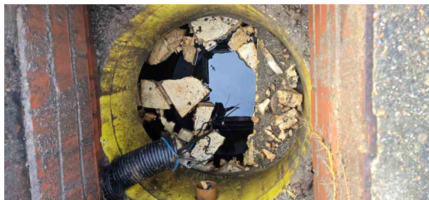
MH23X_b2a02f52-d2a0-40f8-8de7-244e290f80c2_20241125_100934.jpg, 00:00:03, 0.00 m General remark, INTERCEPTOR REQUIRES EMPTYING TO SURVEY
