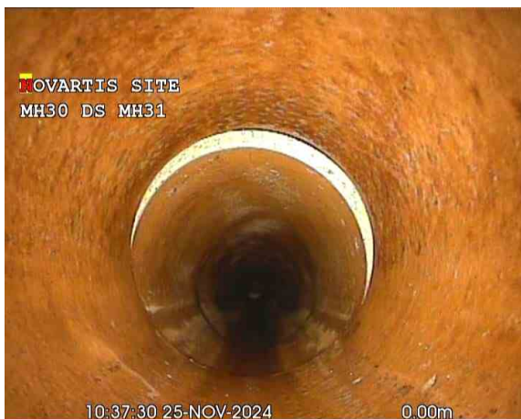
MH30X_be1fa4e2-0bad-4938-8c7d-66491d64b79e_20241125_104944_019.jpg, 00:00:10, 0.28 m Joint displaced, large
