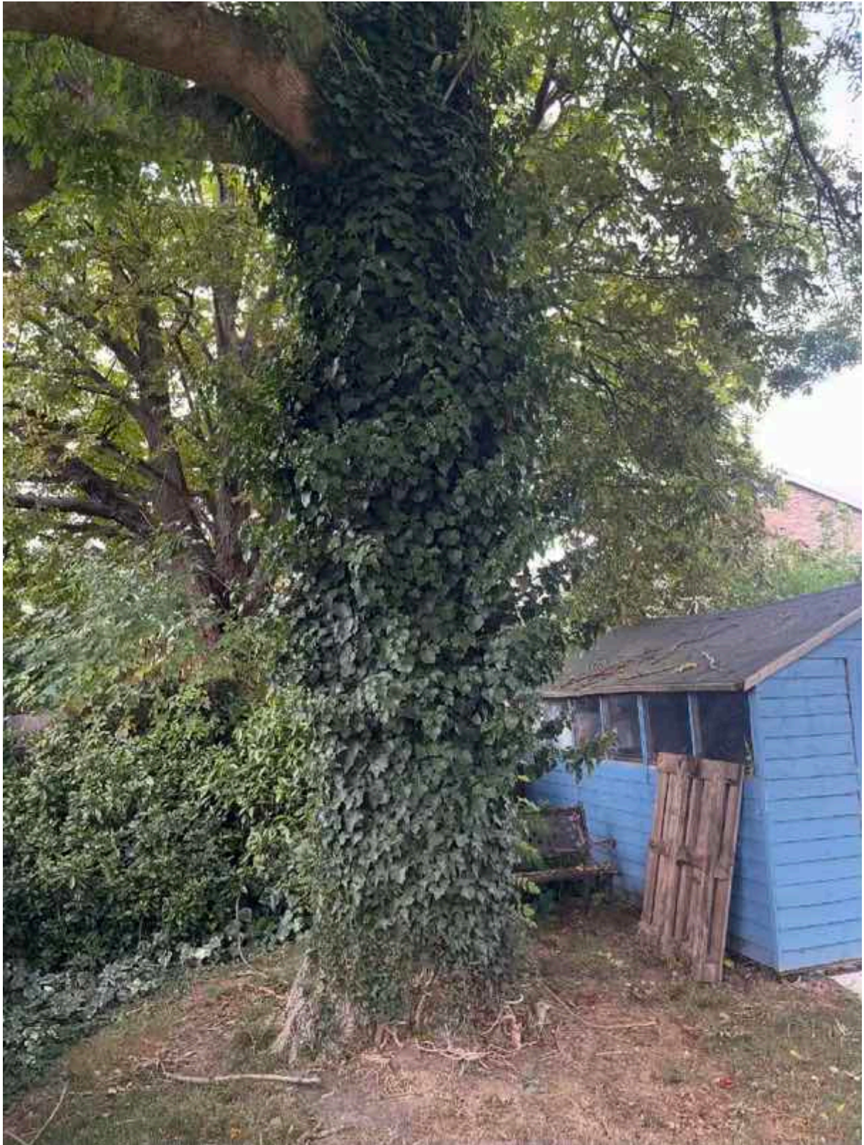
T3 Ash tree - remove ivy and wooden sheds around baser of tree
