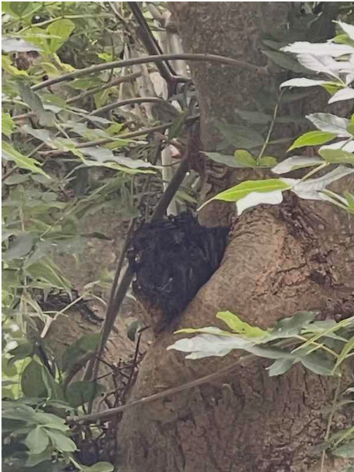
T3 Ash tree - possible fruiting body of Inonotus hispidus to be inspected
