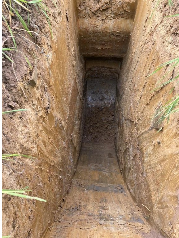
Photo 7 – TP05 prior to reinstatement with seepage visible.
