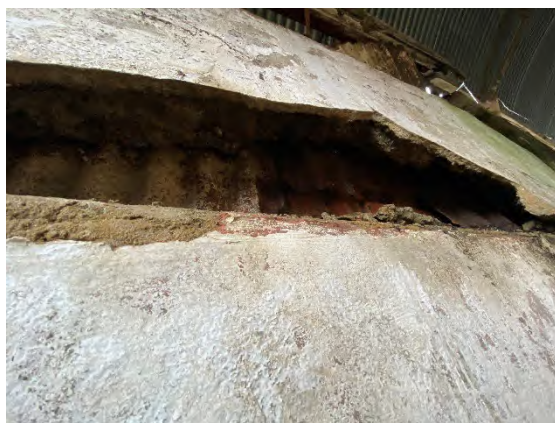
Photograph 2. Crumbled wall forms a dry crevice.
