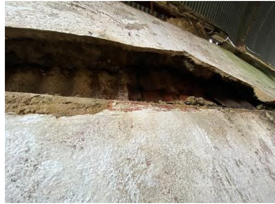
Photograph 2. Crumbled wall forms a dry crevice.
