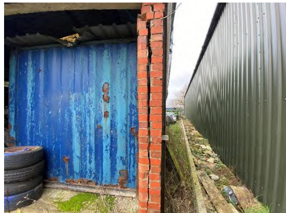
Photograph 6. External wall of B3 forming crack crevice.
