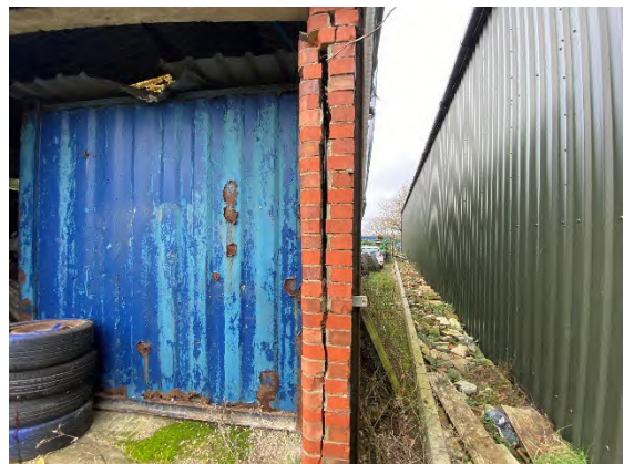
Photograph 6. External wall of B3 forming crack crevice.
