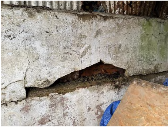
Photograph 1. Interior wall of B3 that has crumbled.
