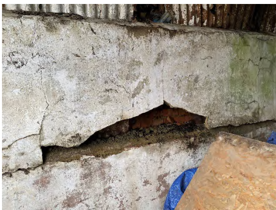
Photograph 1. Interior wall of B3 that has crumbled.
