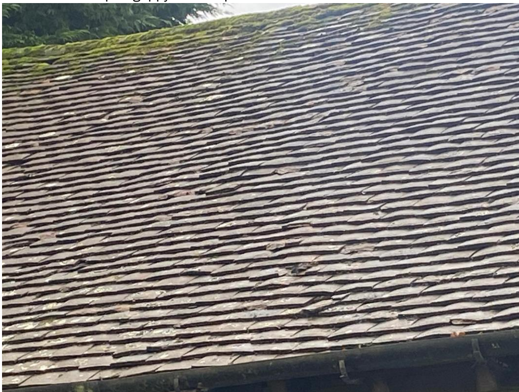
Photo 6 - Closeup of gappy and misplaced tiles.
