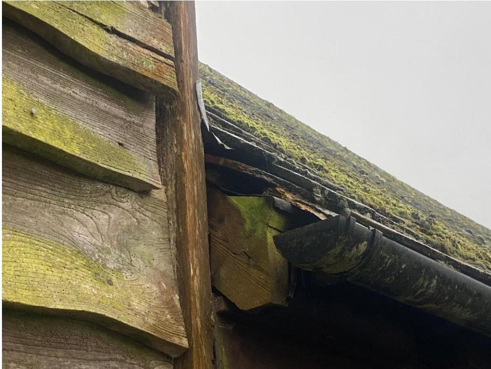
Photo 5 - Detail of gap in western half of barn roof.
