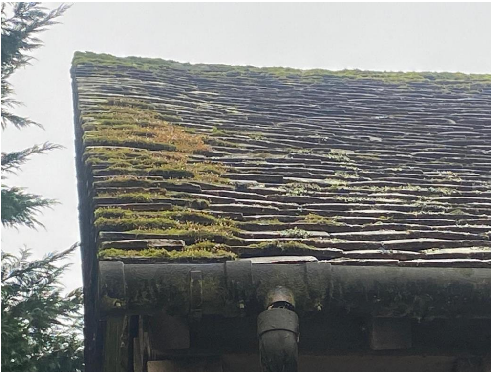
Photo 4 – Area of lifted tile at eastern end of roof.
