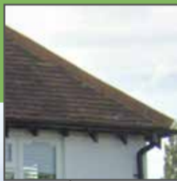
EXPOSED RAFTER FEET
