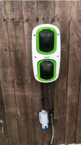
Electric vehicle charging point
