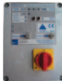
Pump control panel
