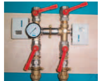
Dual pump switchboard
